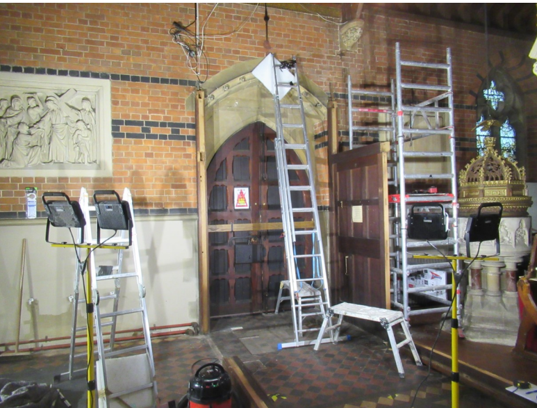
The 'box' is gone. The brackets which would have held a curtain prior to the 'box' are still there. One can be seen just under the corbel.
