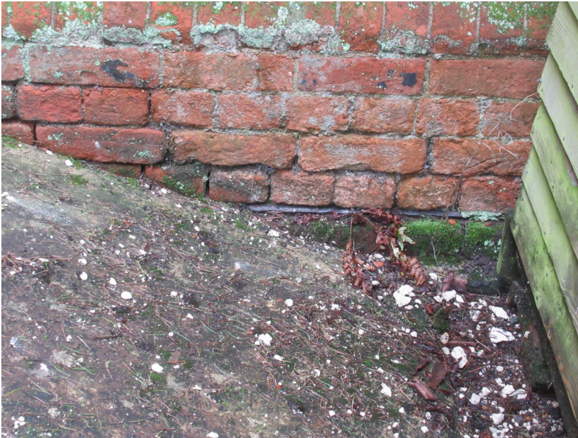
See how the roof of the boiler room is built over the damp proof course of the
