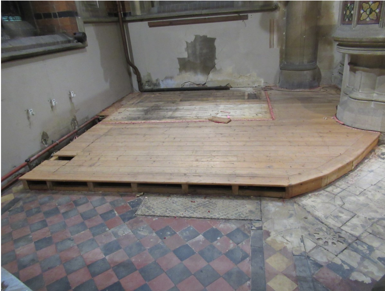
The dais under the side altar. Note the damage to the wall from the damp the other side – see boiler room on page 1.
